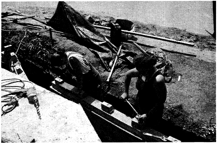
Studio South students Amy Cole and Kelley Hubbard work on the foundation of the Memorial Block.
