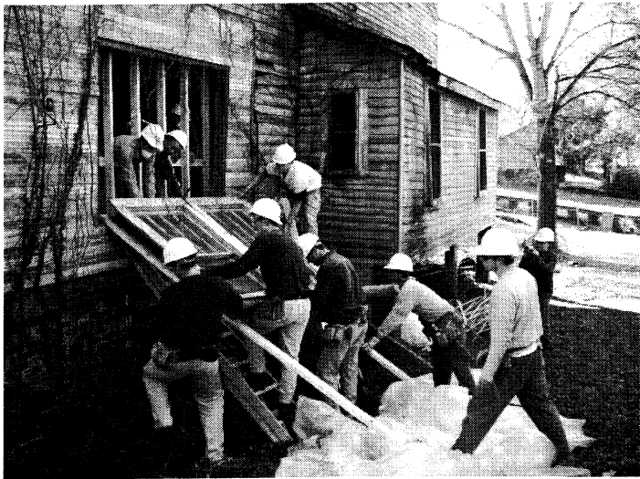
Studio South carefully removes one of the windows to preserve as an artifact of the Keese Barn.
