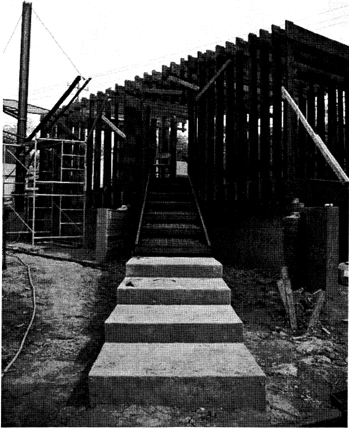
A view of the Memorial Block as the major structure is reaching completion. Reclaimed wood from the Keese Barn form the ribs.
